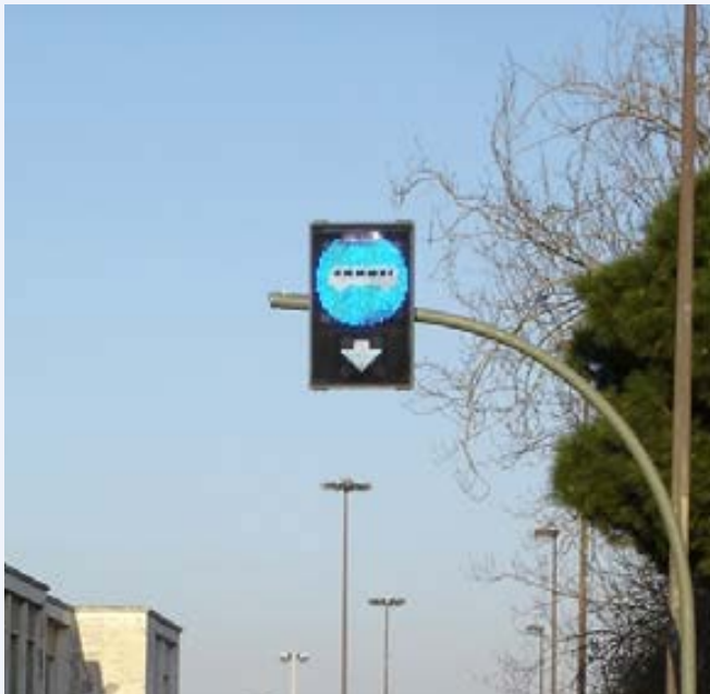
Overhead Lane-Use Control Signals
